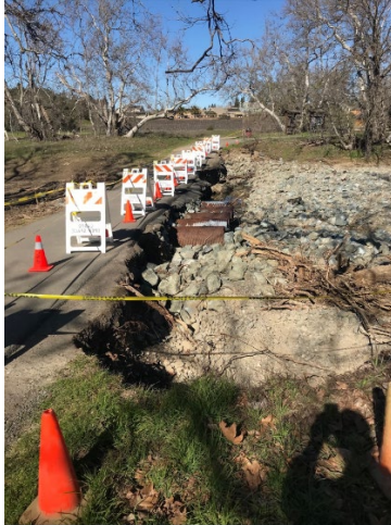
Sycamore Grove Storm Damage
