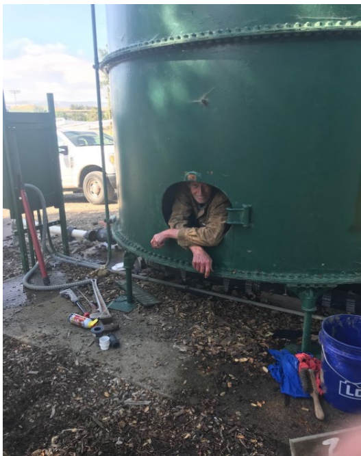
Ernie Rodrigues Water Tank
