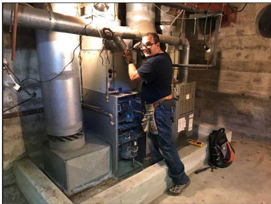
R.E. Merritt Building HVAC
