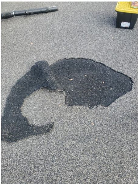
Altamont Creek PIP Before Repair
