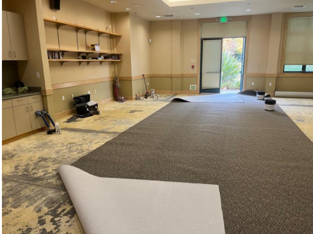
Jackson Floor Damage
